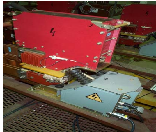
Figure 1: The VAB49-4000 breaker. 256 such switches are required for the LHC main circuits.
