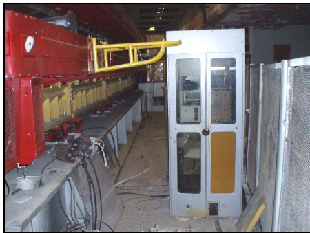
Figure 12: Shelf with a low-level electronics near SS #2 in ring hall of the U70.
