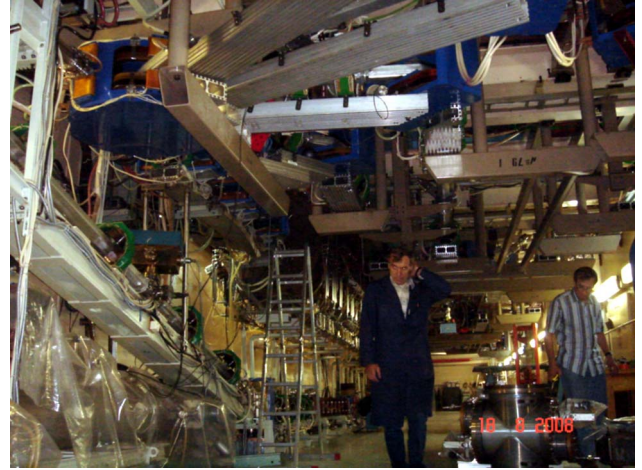
Figure 6: The bends are hanged on the ceiling. Round magnet is at the top left corner, the old terahertz FEL magnetic system is at down-left. Elements of the optical resonator for the second-turn FEL are yet at the floor (down-right corner).
