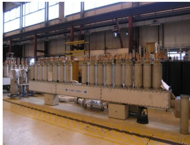
Figure 10: DFBA Cryogenic Electrical Feed Box for LHC.
