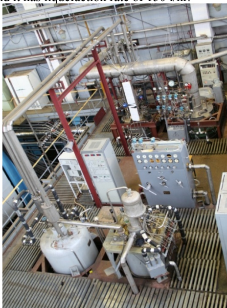
Figure 12: Cryogenic plant and large helium heat exchanger of superfluid refrigerator system of 21 channel.
