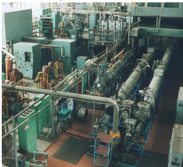
Figure 5: Test facility for study of 6 m length SC magnets and string of magnets. 120 g/s forced helium flow.
