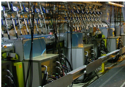
Figure 2: Kickers and amplifiers in the LHC tunnel.
