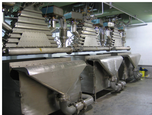
Fig.7. Irradiation hall for waste water treatment with ELV-12 accelerator
