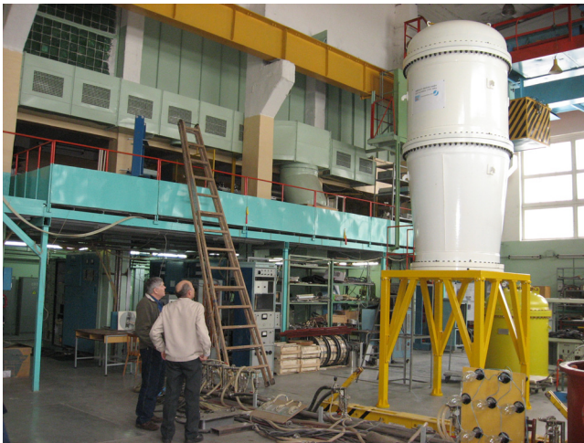
Figure 5: High voltage vessel in BINP Novosibirsk.
