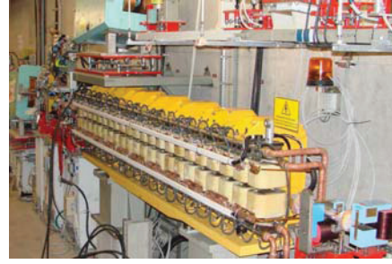
Figure 4: FLASH far infrared undulator constructed by JINR.
