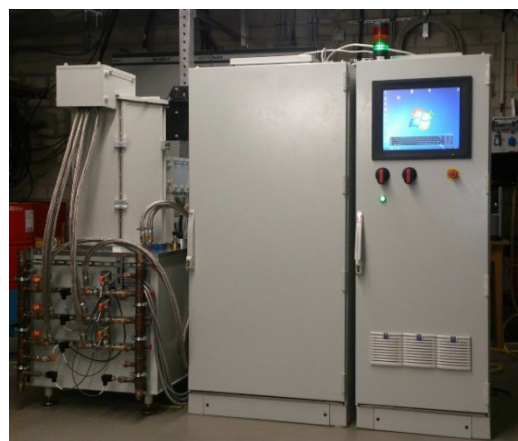
Figure 7: 130 kV modulator with pulse transformer.
