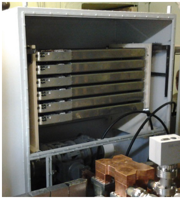
Figure 2: Direct switch solid-state 60 kV modulator.
