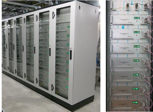
Figure 5: Racks with power supplies: with redundancy system at XFEL (left) and the burn in rack with the measurements crate (right).
