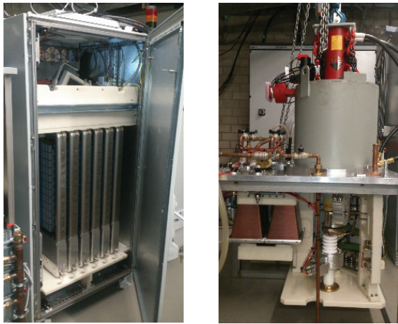
Figure 5: Modulator and RF generator of the TDS INJ.
