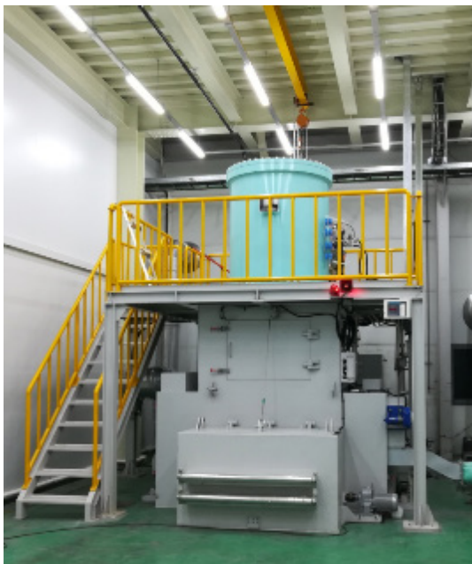
Figure 8: ELV -0.5 accelerator in local steel shielding in Bar Flex Company (Korea), 2018.
