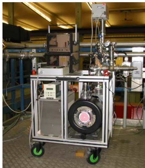
Figure 1: Oil-free pump station as used at the TESLA Test Facility.
