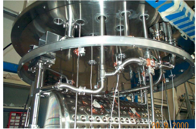
Fig. 8: The cryostat top flange after maintenance: in the centre the newly installed cryogenic valve can be seen.
