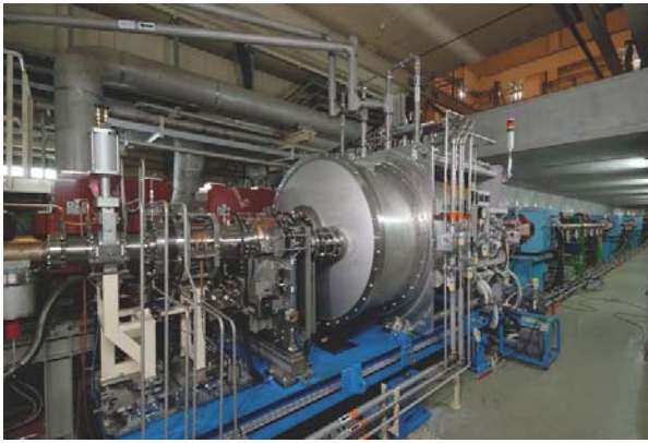
Figure 10: KEKB crab cavity for HER installed in KEKB
