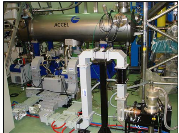
Figure 5: ERLP Cryomodule with RF waveguides
