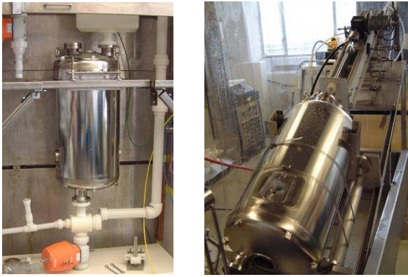
Figure 5: Final BCP following installation of liquid helium tank and coupling ports (left); high pressure water rinse (right).
