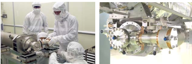
Figure 17: Installation of an input coupler (Left) and an assembled cavity mounted on 2 K gas return pipe (Right).
