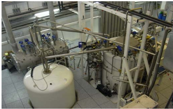
Figure 4 : The cryogenic area in the technical gallery
