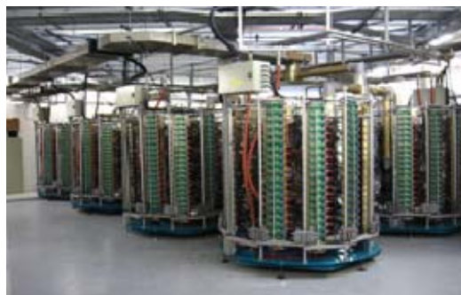
Figure 2 : Amplifiers 1 and 2 in the SR RF room
