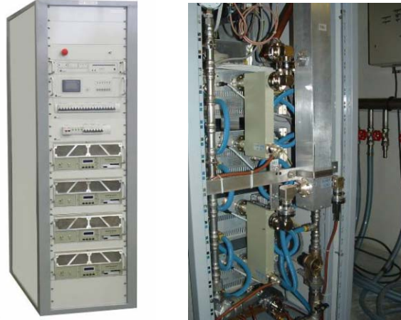
Figure 9: 10 kW cabinet and 6 and 10 kW hybrid combiners.
