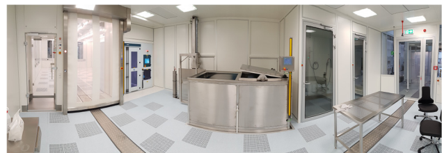
Figure 1: Fisheye perspective of CR 1 (ISO-6). In the middle part the US and C-rinse baths are shown, on the left: Personnel air lock, roll-up door and part of the HPR.
