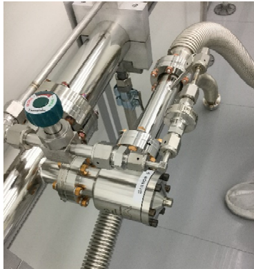
Figure 1: Nitrogen purging and evacuation merges at the beginning of the corrugated vacuum hose.
