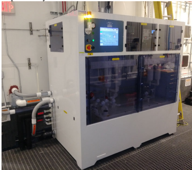
Figure 3: Remote electrolyte sump unit.
