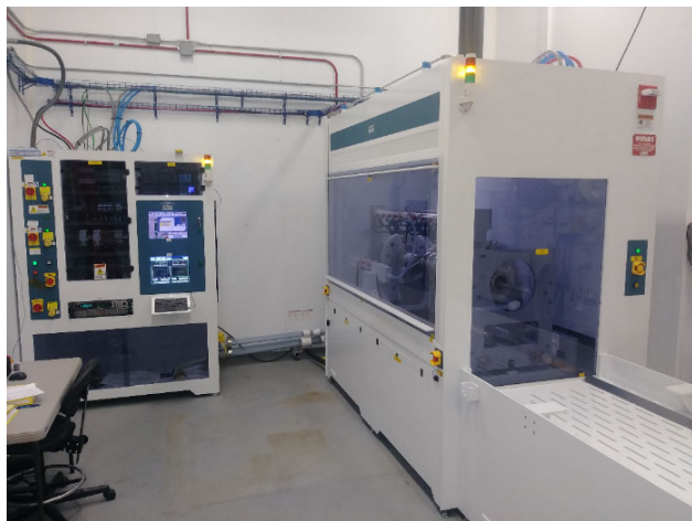
Figure 1: New JLab cavity EP system.
