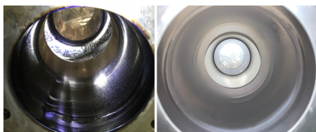
Figure 5: Left: Cavity inner surface before coating. Right: Cavity inner surface after coating.
