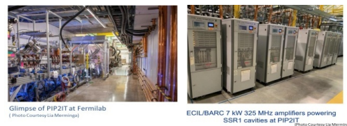
Figure 15: 325 MHz solid state amplifiers for PIP-II IT supplied by BARC.
