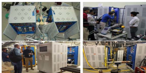
Figure 10: Upper photos acceptance testing of first 650 MHz SSA prototype at RRCAT. Lower photos the amplifier shipped to Fermilab, assembled and tested for rated power.
