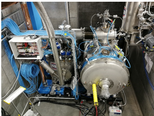
Figure 2: One ESS DSR spoke cryomodule at FREIA.
