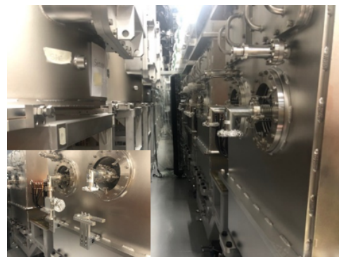
Figure 2: Installation of HWR cryomodule in the tunnel. DC-bias tee is assembled with the RF coupler in small picture.
