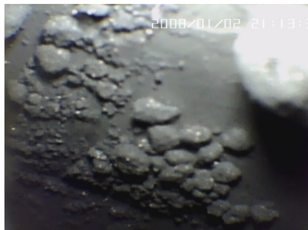
Figure 2: Niobium oxide dust at the bottom of the WiFEL cavity, as seen through the cavity port (top). A close up view of the contamination, seen through a flexible borescope inserted into the cavity prior to cleaning (bottom).
